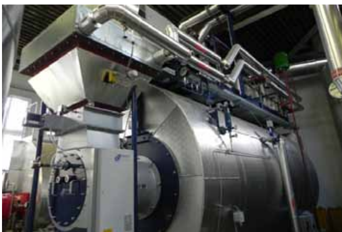
Steam generator plant with modulating natural gas forced air burner and air preheater
